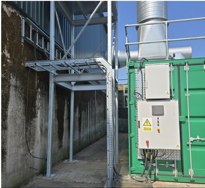
Industrial containment and cabling
